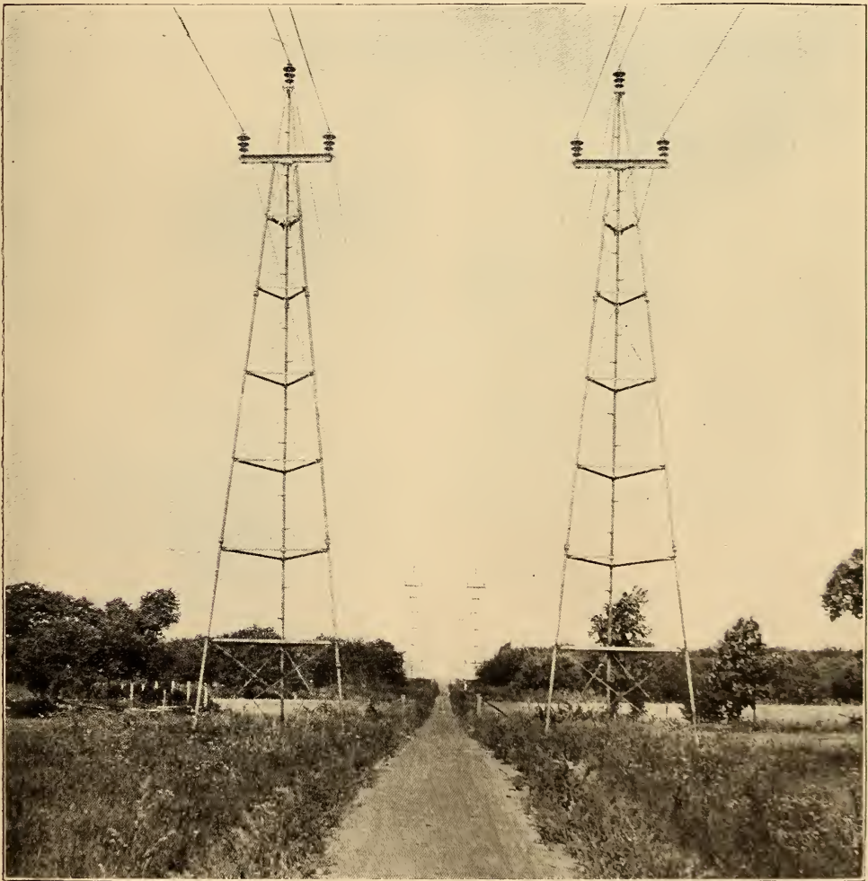
FIG. 2. TRIPOD TOWERS FOR TRANSMISSION LINES.
