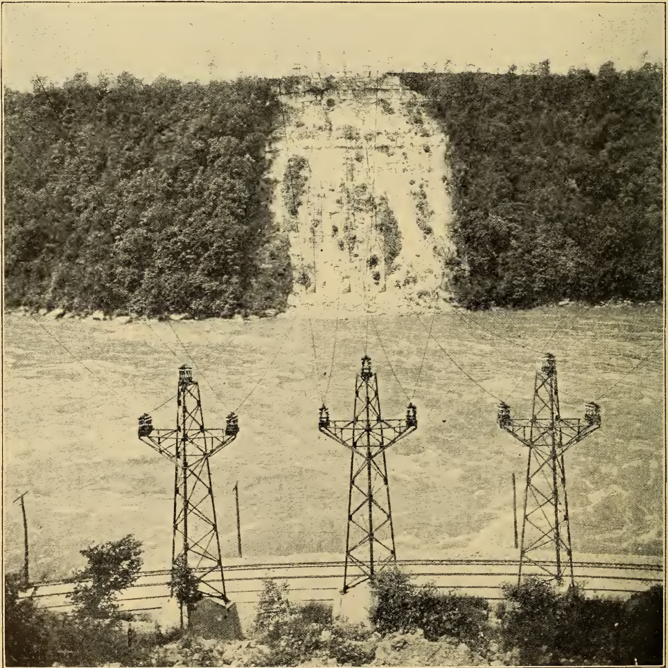
FIG. 1. ELECTRIC CABLES ACROSS NIAGARA RIVER.
