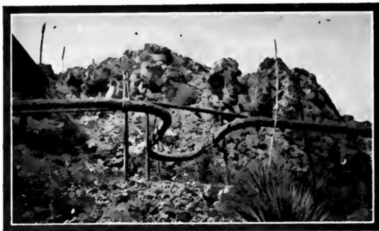
Expansion and Contraction, as Well as Vibration, May be Taken Care of by a Loop in the Piping.
