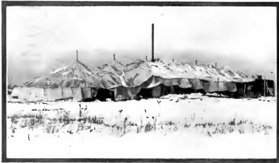
In Order to Carry On the Work of Erecting a Building During the Winter, a Cleveland Contractor Used a Large Tent.
