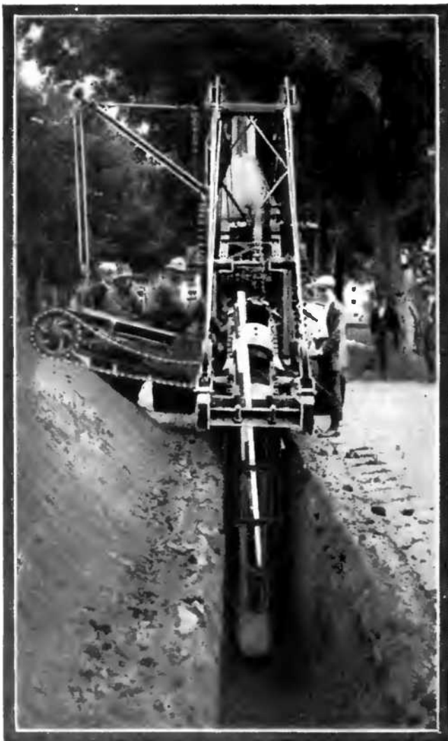
A New Trench-Digging Machine that Operates at the Rate of Four Feet of Trench Five Feet Deep and Two Feet Wide Per Minute.
