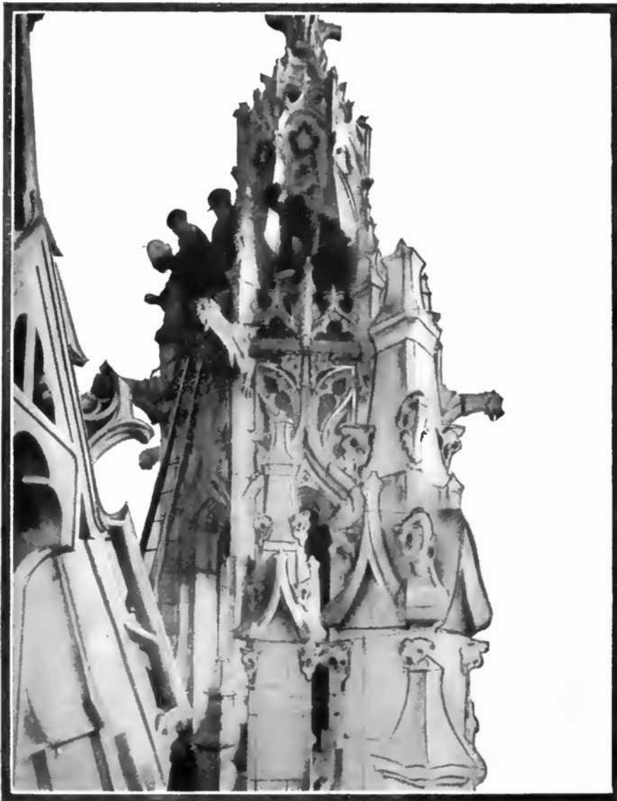
The Electricians who Placed the Electric Lamps and Ran the Conduit had a Perilous Task Before them, Often Working on Uncertain Foot-holds Many Hundred Feet Above the Street.
