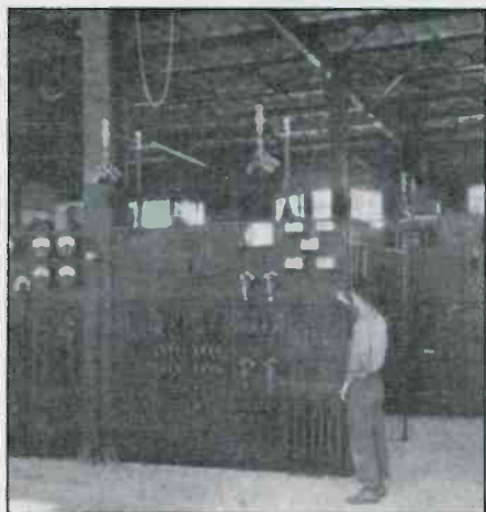
In 1920, the main antenna relay switchboard looked like this. It was remotely controlled from New York City, but could be manually controlled locally if necessary.
