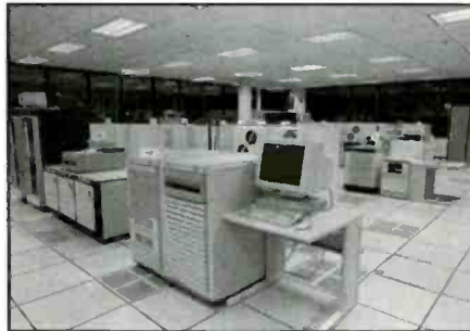
The data floor of the USCG Operations System Center in Martinsburg, West Virginia which includes the AMVER Center (USCG Photo).
