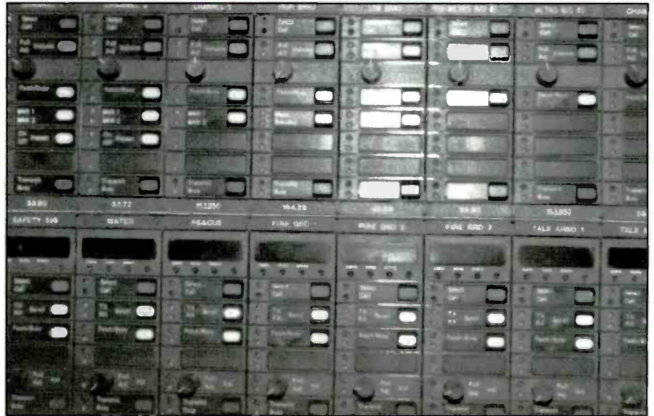
Closeup of Motorola talk group control modules at the Cleveland Fire Department dispatch center. (Photo by Stephen Bellamy)
