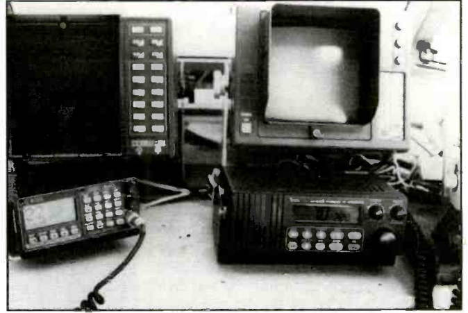
Emergency fireboat with twin DSC (Digital Selective Calling) radios onboard.
