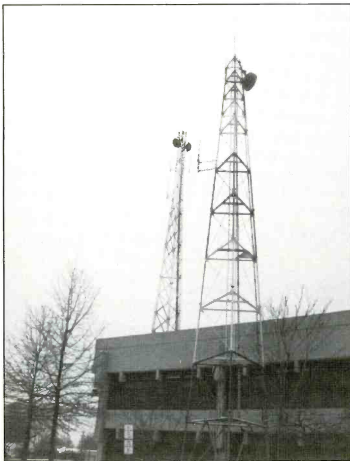
The tower in the background is one of the eight 800 MHz trunked, simulcast system towers. Note the microwave dishes for system linking. (Photo by Stephen Bellamy)
