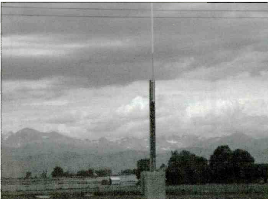
Transmitter control boxes and antenna base.
