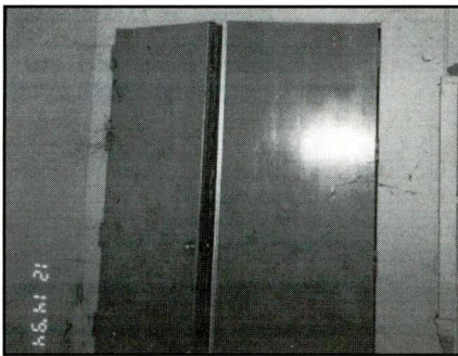
Massive door from underground bay to internal ramp running up to the maintenance bay.
