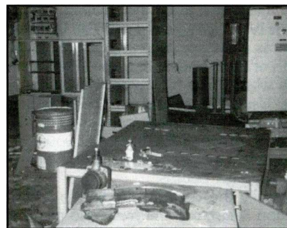
Tranmitter/Receiver (?) room with racks and shells of equipment.
