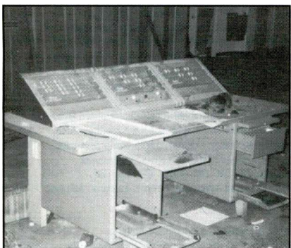
Antenna switching console in underground bay. Computer (?) racks can be seen in background.
