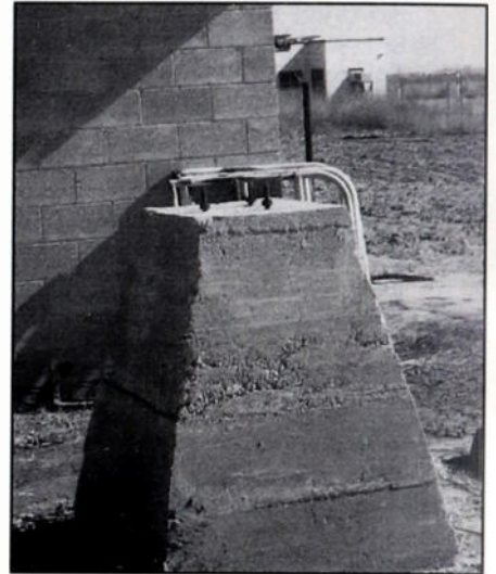
Existing remains of the concrete base that once supported the KYOR tower at the abandoned site. (Photo provided by Jan Lowry of Broadcast Pro-File, Hollywood, Calif.)
