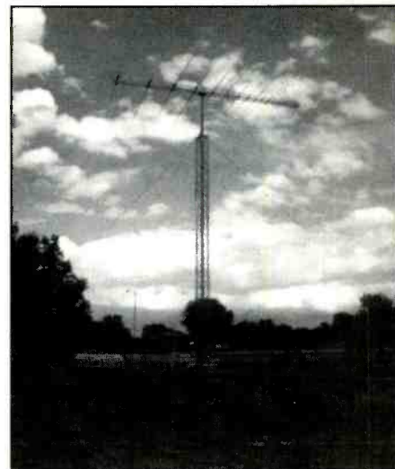
Log-Periodic SW antenna at the FAA Longmont, CO Air Traffic Control Facility. Photo provided by Patrick Griffith, CO.
