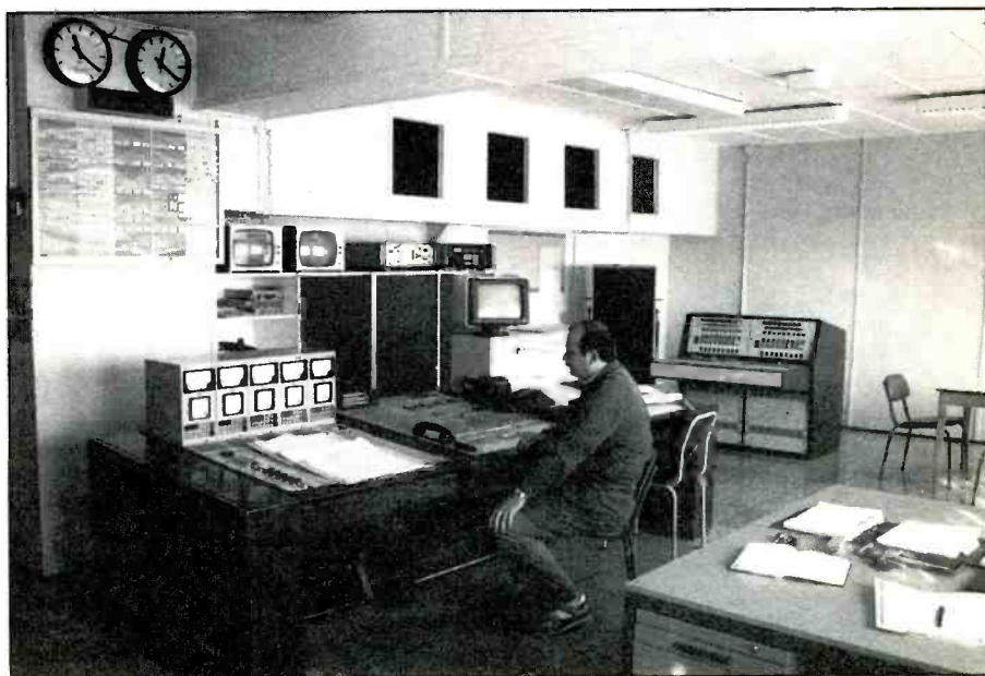
Master Control room for the Radio Deutsche Welle Nauen transmitters.
