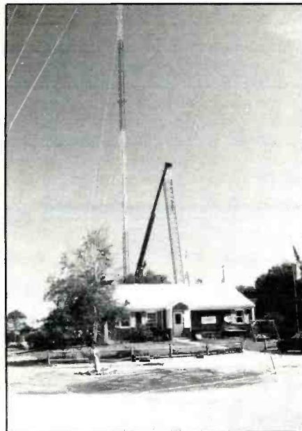
The WCIB tower under construction is the short one at the right.
