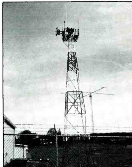
View of several FAA antennas at Martinsburg, WV. (Photo by Charlie MaCatee, WV.)
