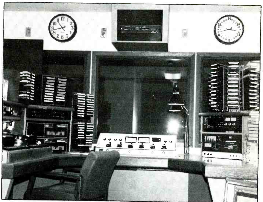
Staff engineer Tim Coucke took this photo of the KNLS control room. The Optomod HF audio processor unit is just to the right of the control board.
