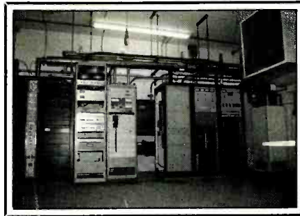
At WAPL-FM (l. to r.) we see a new BE 30 kW transmitter, two STL and control racks, a 25 kW Collins stand-by transmitter, a 3" coax switch, and 50 kW dummy load. (Courtesy Mike W. Flenz, WB9ANR.)
