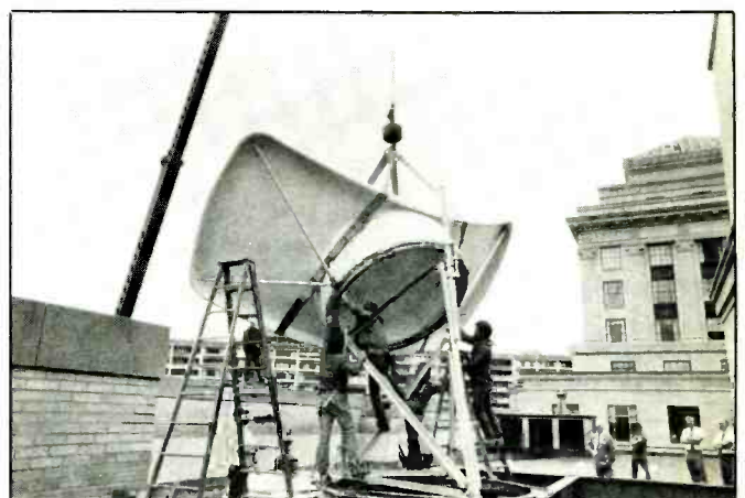
Installation of the satellite up-link on the roof of the Christian Science broadcast center. This dish transmits signals to Westar III.
