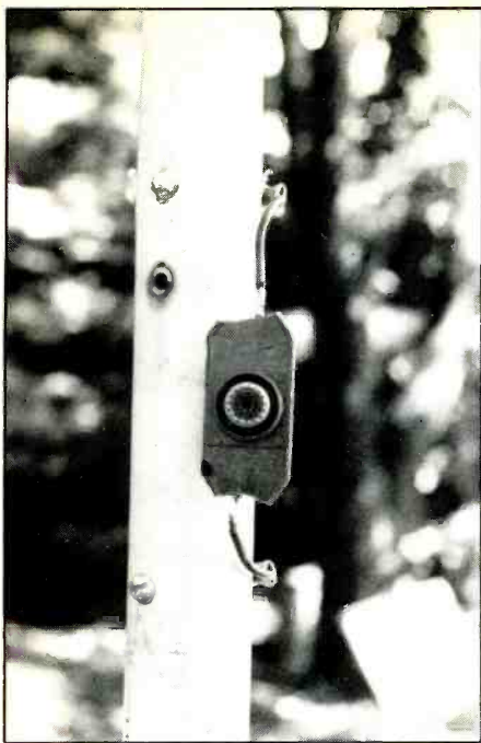
Figure 3: Dipole-to-coax line connector attached between bottom of radiator and bolt to which radials are to be connected.
