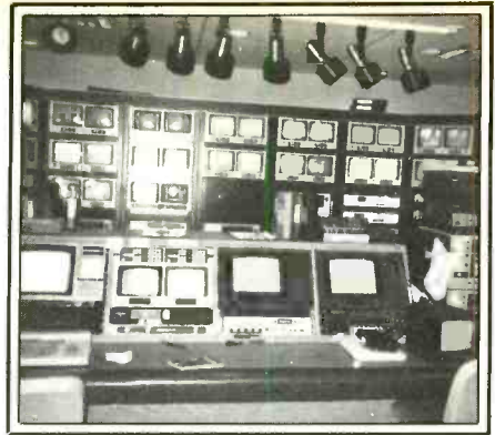
The computerized master control center in Indianapolis.
