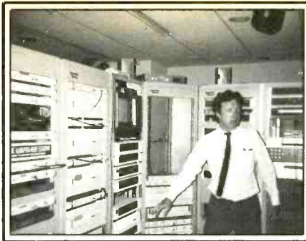
Mike Jones, Special projects Manager for American Cablevision, points out some of the features of the equipment at the Indianapolis facility.
