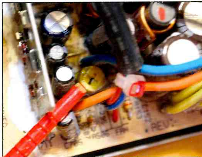
Photo D. This close-up image points to the location of the voltage adjustment in this switching supply.
