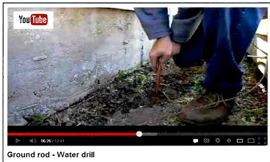
Photo B. This video gives tips on turning your ground rod into a "water drill," taking the pain and strain out of driving 8-foot-long copper pipe into the earth. Visit: < http://bit.ly/ZRobQI >. (Internet screen grab)
