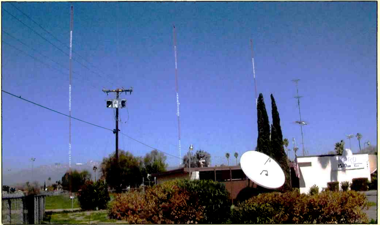
Most AM directional arrays are tough to photograph in their entirety and with the related studio/transmitter building in full view. Pop'Comm Editor Richard Fisher managed to squeeze 3/4 of the 1570-kHz version of KPRO antenna system — plus some of the shack — in this colorful shot.
