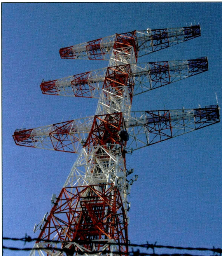
Photo A. The unique Armstrong Tower is designed with three cross arms to maximize horizontal and vertical space for antennas. (Courtesy of WPC1CAT)
