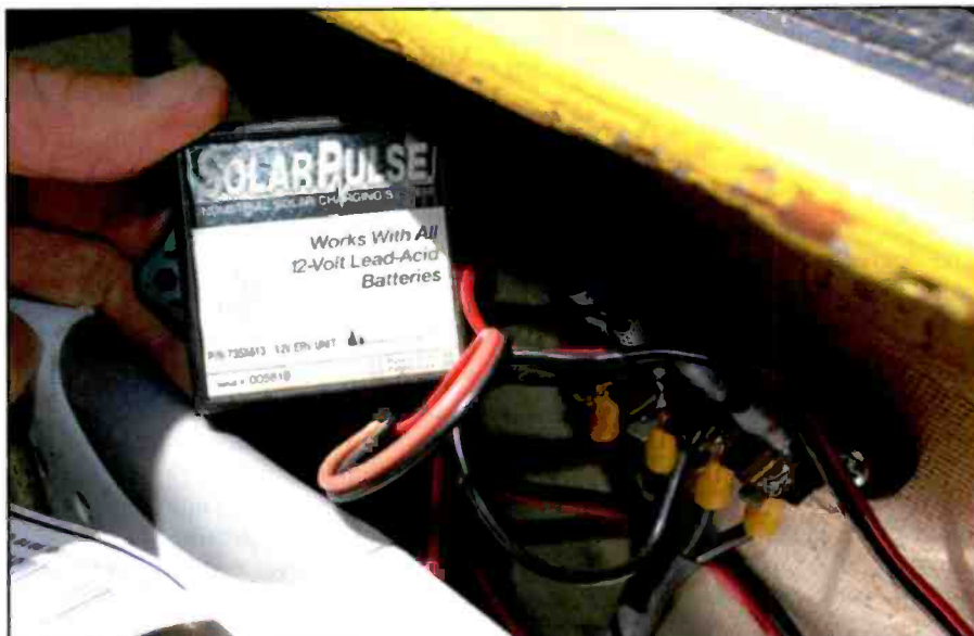
Photo E. Carefully inspect how the reserve source of energy (RSE) is getting its battery recharged.
