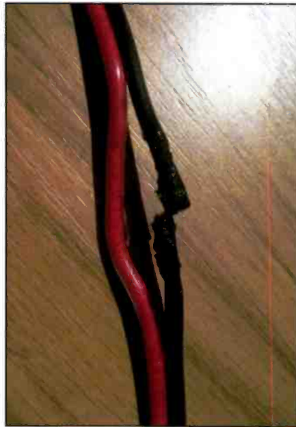
Photo G. Carefully inspect VHF radio power leads — in this installation, stray ground currents have melted the DC negative lead. Both red and black DC leads will need to be replaced.
