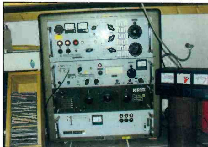
Equipment used at Black Arrow Radio. (Courtesy of Rich D'Angelo)
