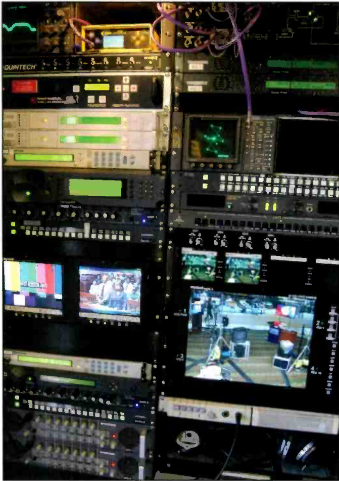
Photo L. A WFXT equipment rack shows the complexities of putting together live remote coverage, as Fox 25 Boston did during the New Hampshire primary.
