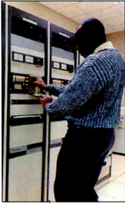
Transmitter control panels at WEWN, Birmingham. (Thanks Charles Maxant, West Virginia)
