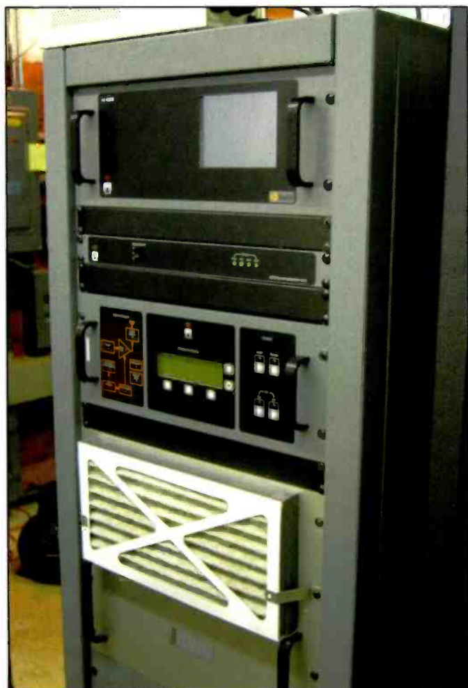
The station's Nautel J1000 transmitter outfitted with HD digital and GPS synchronization units.
