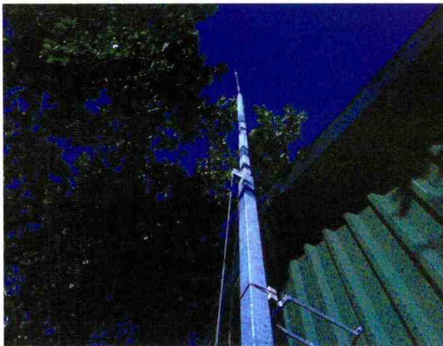
Photo B. The vertical antenna of Radio Quintas mounted against a steel shed.
