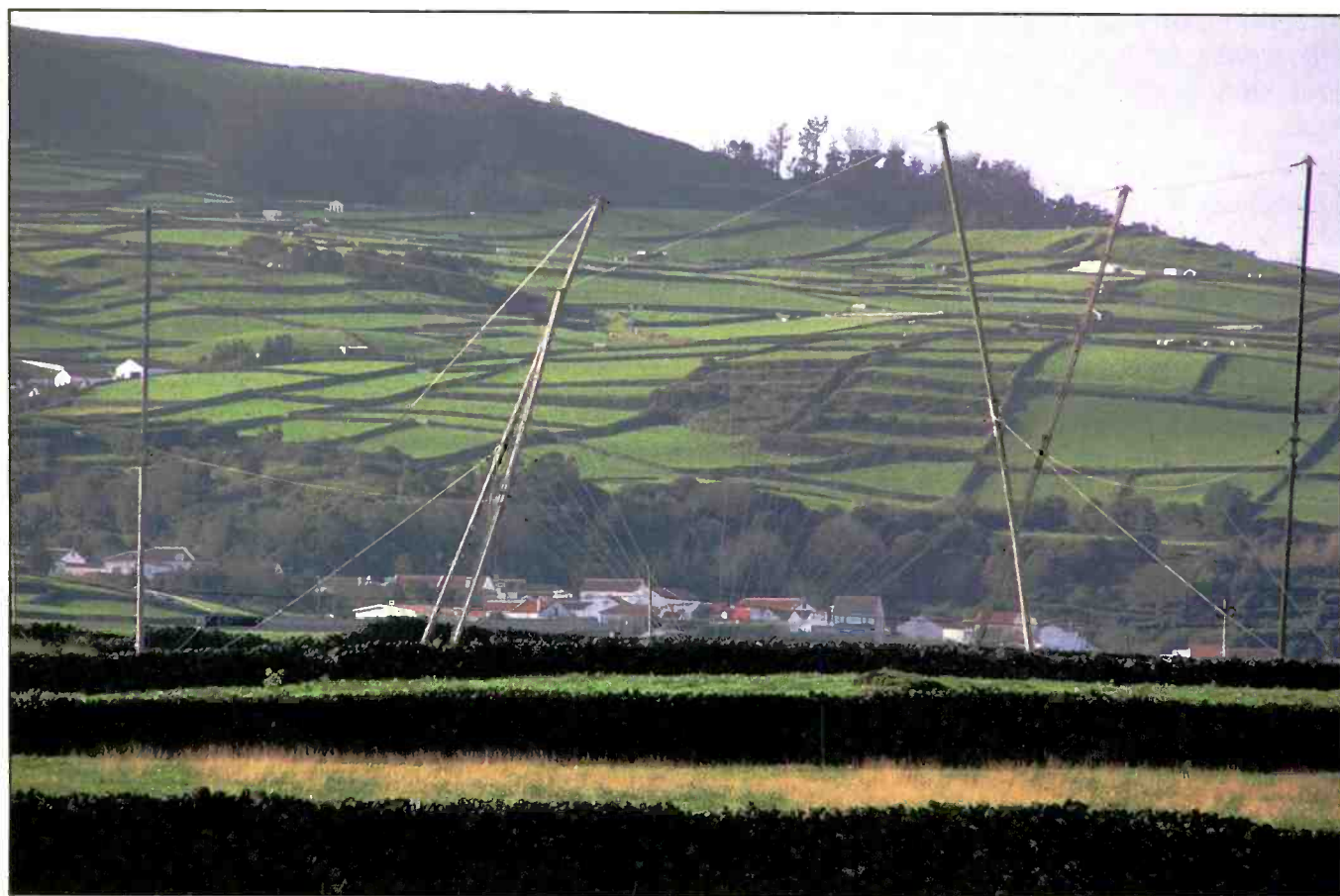
Photo A. The antenna farm at the Lajes HF-GCS station. (USAF Photo)
