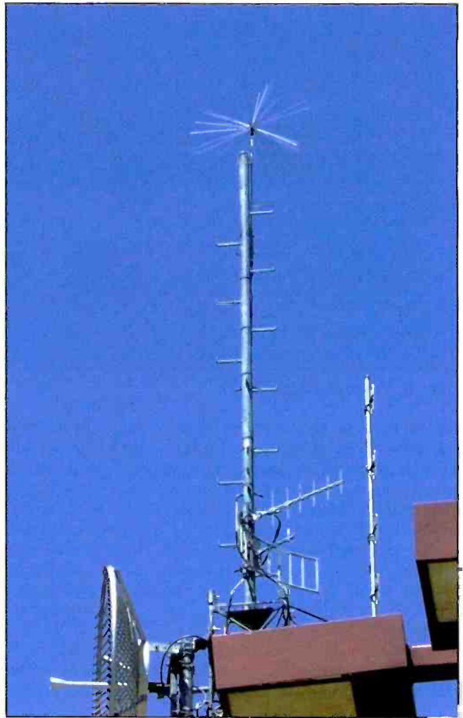
Photo D. Commercial tower with lighting dissipater.
