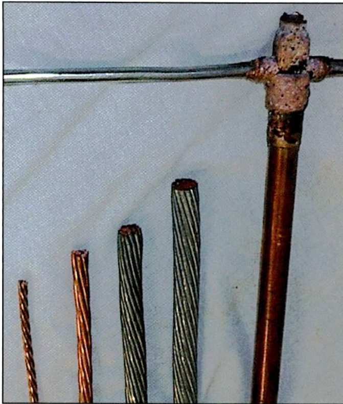
Close up of a completed "Cadweld" exothermic weld of a #2 solid copper wire to the top of a 5/8-inch-thick ground rod and examples of ground wire relative sizes. From left, #6 stranded copper ground wire, #2 copper wire, #2/0 wire, #1/0 wire, Cadwelded 5/8-inch ground rod.
