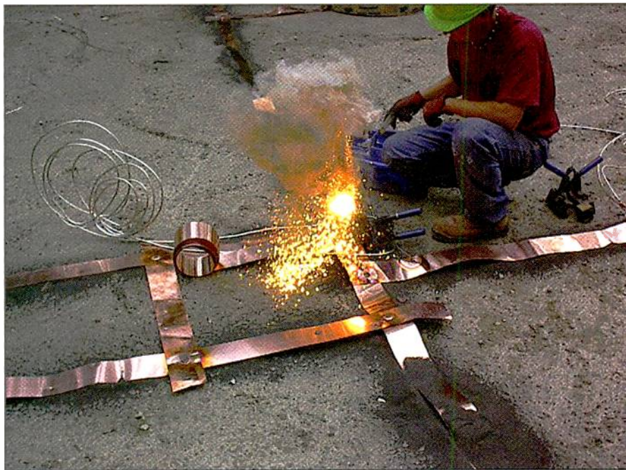
A worker "Cadwelding" (see text) #2 solid copper wire with 4-inch-wide flat copper strap. The dark material around the copper strap is Harger "ground enhancement."
