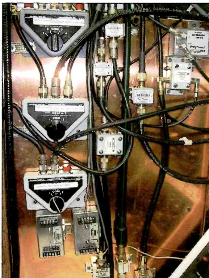
This photo, taken in the author’s hamshack, shows a “single point ground” panel with various coax switches that put unused antennas to ground, along with several brands of lightning arrestors. The copper sheet is “bonded” with the outdoor ground system with a 6 inch wide copper strap. The sheet is .022 inch thick copper screwed to a 3/4 inch thick plywood panel.
