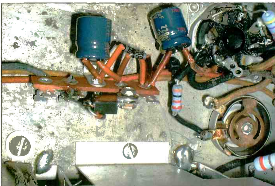
Photo H. The original battery pack may have been state-of-the-art 60 years ago, but the problem-prone dry cells are now easily replaced by a small handful of modern solid-state components. Note that I tack-soldered the shields between the band-switch sections directly to chassis to ensure stability.
