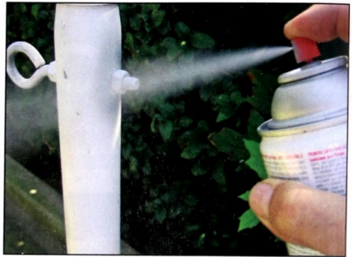
Photo E. Apply a coat of primer paint to all exposed hardware, then finish with exterior enamel once the primer coat is dry.
