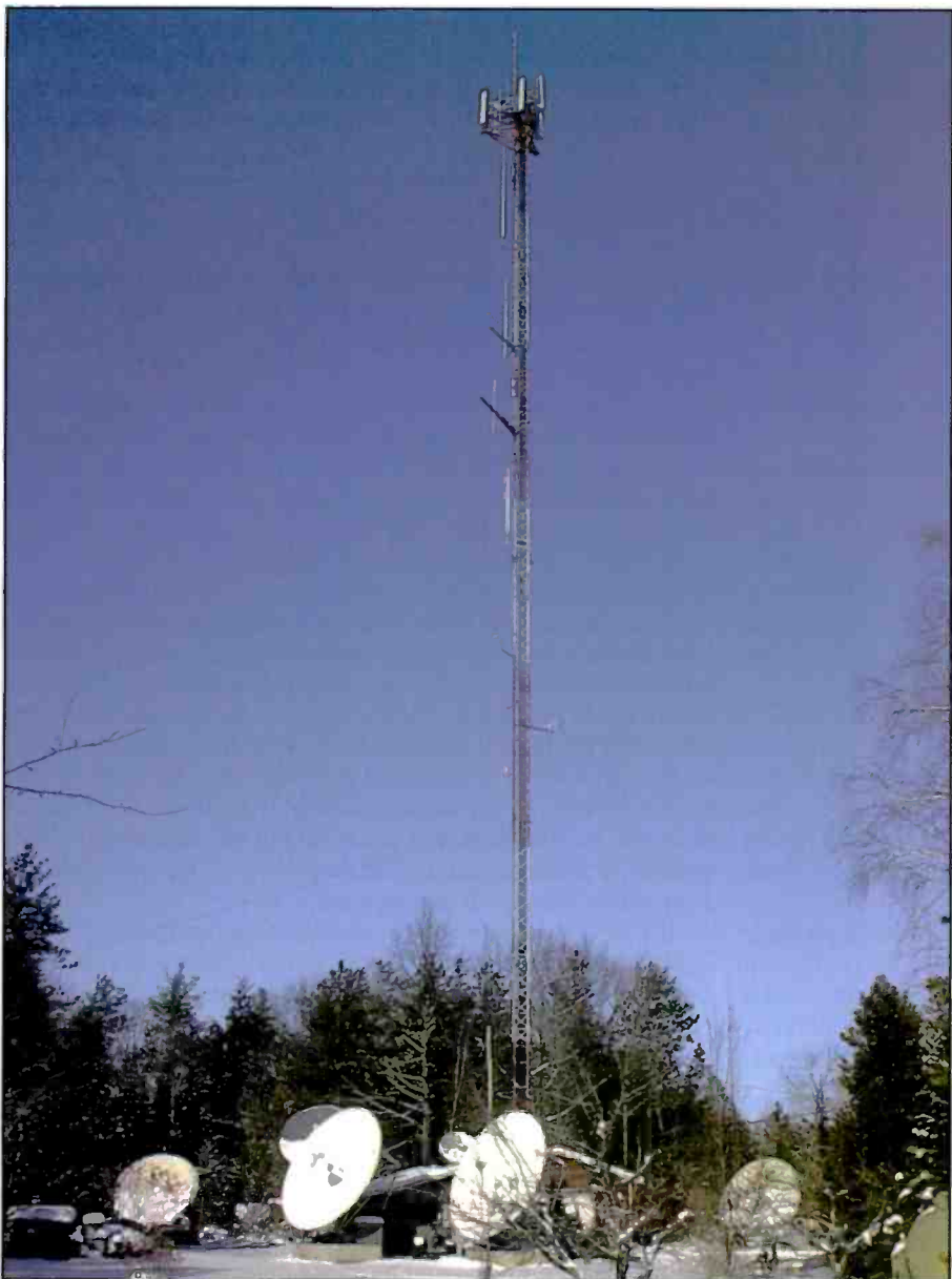
Or think tall...A PiRod 200-foot commercial tower recycled to ham radio use when the cable company went to fiber optics. This photo also shows some satellite dish antennas.
