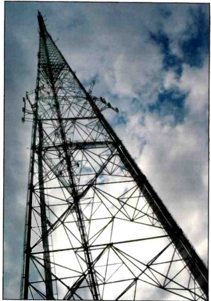
There's a wealth of things to listen to no matter where you are. Dozens, maybe hundreds, of users can share a large tower like this one in every band available. Note the antennas on stand-offs mounted about halfway up the legs.
