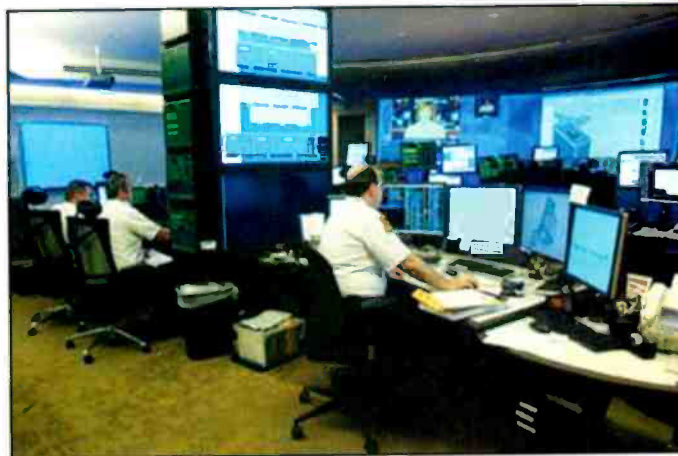
A look inside FDNY's new $17.5 million radio communications center, which opened in September 2006. (Courtesy City of New York)
