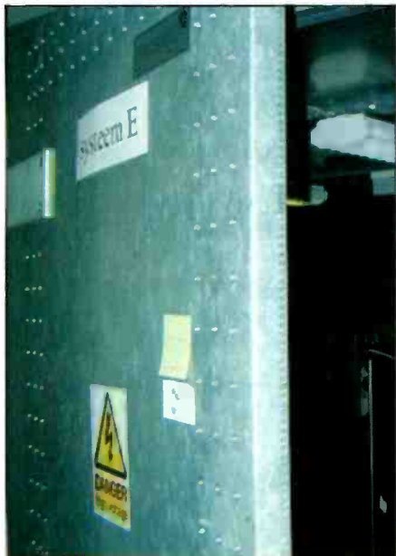
Here's a Faraday shield that encloses an entire room. Note the connection points along the edge of the door that ensure a complete electrical connection of all surfaces. No matter the size of the "box," the same principles apply. What you build will be just as effective as the professional model, as long as you take your time and follow the instructions provided in the column.
