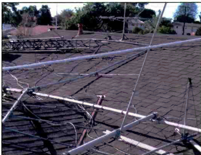
Southern California twister damage on the roof.
