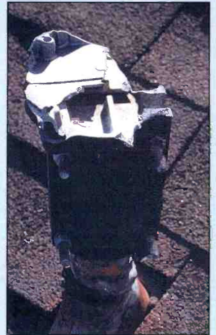
After the tornado...rotator failure!
