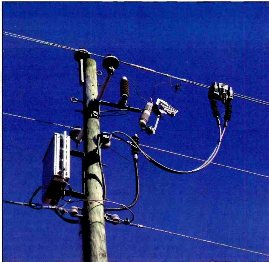
Here's a photo of a pole-mounted "Extractor," made by Amperion and used in the Progress Energy trial near Raleigh, North Carolina. The vertical "rod" or bar attached to the side of the cabinet is an 802.11b "WiFi" antenna. This Extractor picks the data off the BPL signal and converts it to WiFi for a hop across the street where it's re-injected into the underground power line as BPL to be distributed around the neighborhood. The Extractor is coupled to the power line by induction at those clamps hanging on the line on the right side of the picture. There is no physical, electrical connection to the line. Amperion says that the hardware can be attached to a live power line with normal precautions.
