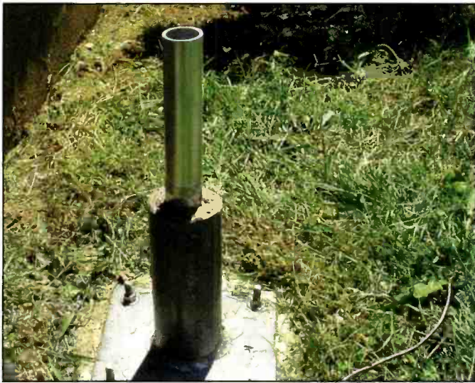
The mounting pole inserted in the small flagpole base. Cement was also placed around the mounting pole.
