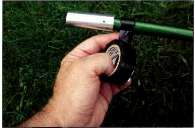
All fiberglass pole joints are securely taped with the provided electrical tape, then covered with a special self-sealing tape. This photo shows the tip of the antenna being prepared for the vent cap.
