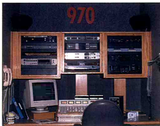
Racks of equipment and patch bays in the Portland Radio Group engineering command center.
