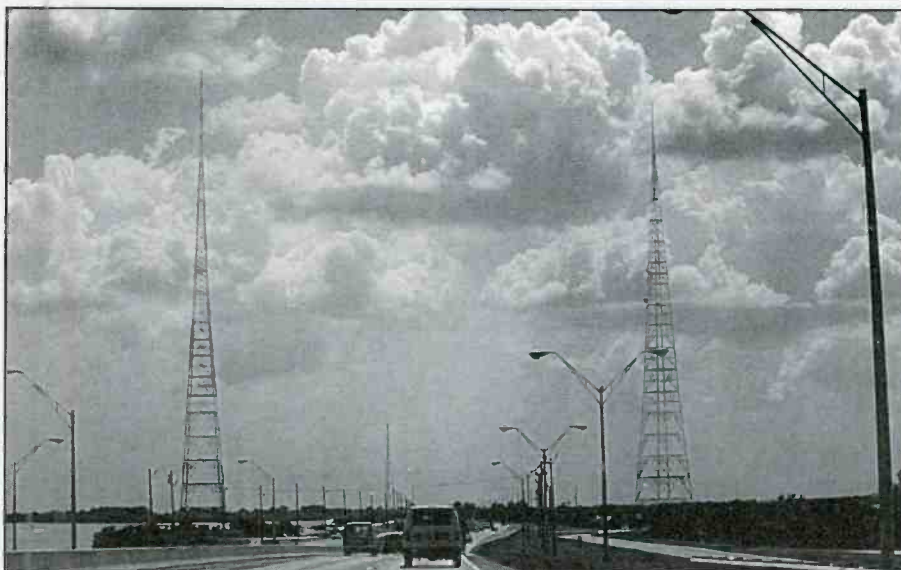
The two antennas that produce the directional pattern for 620 AM in St. Petersburg, Florida, are dissected by Route 92.
