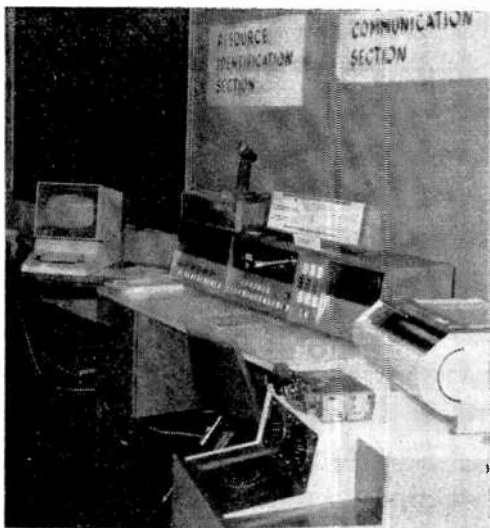
Communications Center for Project 20/20 is a model of its type. Computer display provides information as to proper agency to notify in emergencies.
