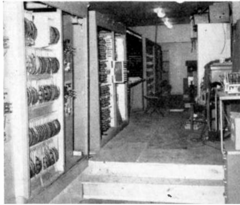
The 1103, in two rows of cabinets like these, takes up almost all the space in Al Domin's parts store.
