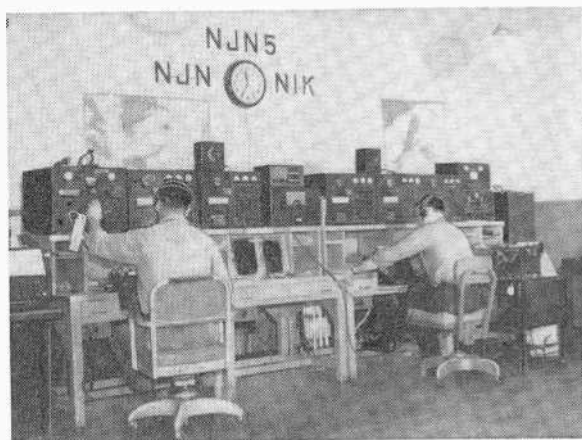
A typical USCG shore station radio installation is the International Ice Patrol HQ at Argentia, Newfoundland.
