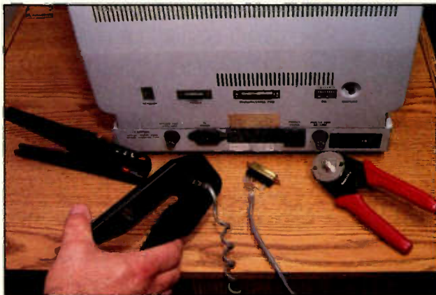
In this application, an 8-position silver satin line cord must be stripped and, depending on the hardware, a DB-25 or RJ-45 connector must be installed.
