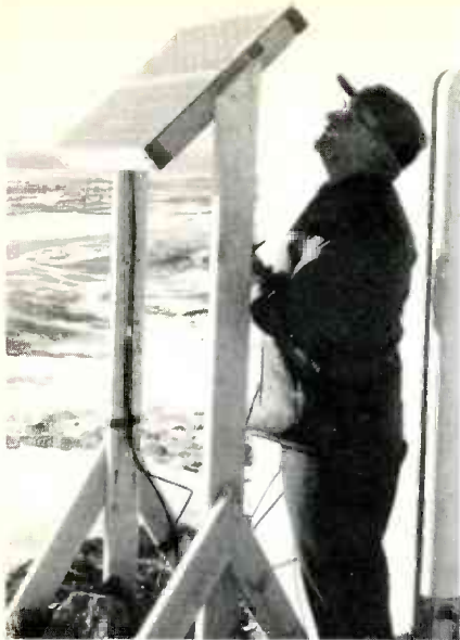
A 4-watt 32-volt solar-cell panel on Johnny Moore Mountain supplies DC power to operate the translator, and to keep the storage batteries charged.
