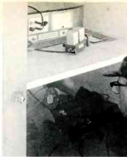
On the top shelf of the discarded refrigerator (used to give protection against the weather) are the Channels 4/8 translator, and a Channel 8 bandpass filter, while on the bottom shelf is the bank of lead-calcium-alloy storage batteries that furnish DC power at night and during overcast days. John Gresham is shown checking the batteries.
