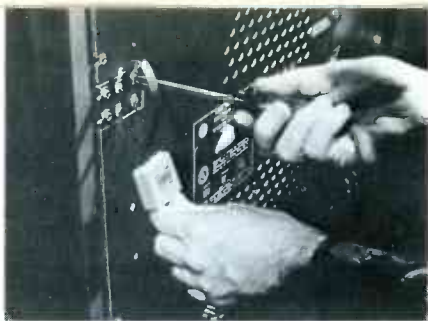
Fig. 15 Most TV receivers have 300-ohm input impedance, and so require a matching transformer between the terminals and the coax cable. For all-channel installations where the receiver has separate UHF and VHF terminals, the matching transformer should be a frequency-splitting type, as shown.
