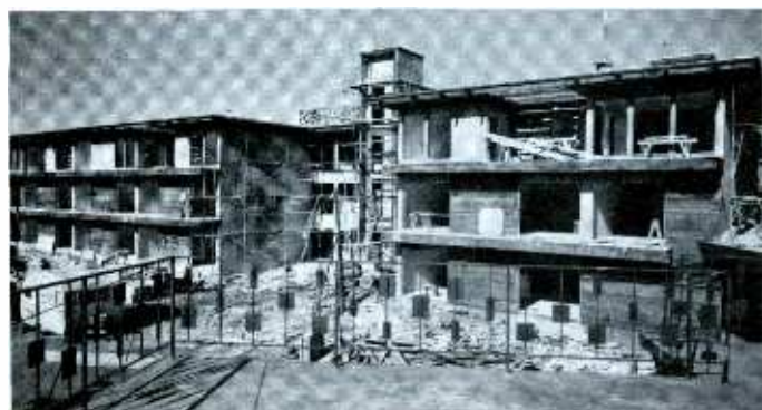
Downey, California — The Tahitian Village, under construction, has 10 buildings ranging from 14 to 48 units; a total of 200 outlets when completed. Wizard systems are used throughout.
