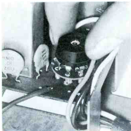
Fig. 7. Installing a socket by inserting it into the risers of the old one, wired as shown in Fig. 5B. Some suitable transformers are listed in Table I.
