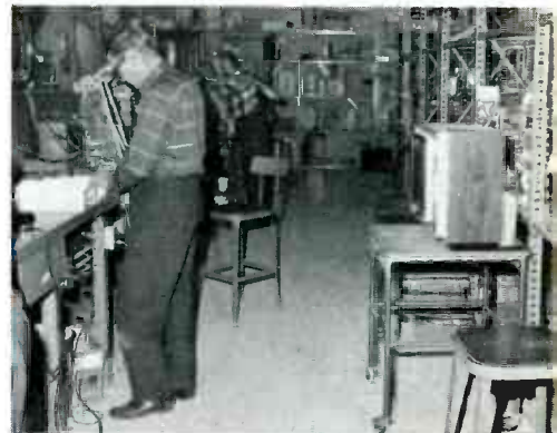
WORK BENCHES are steps away from the 'in' rack.
