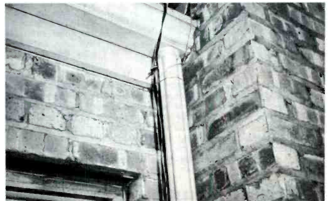
Fig. 13. Improper Method of Running and Connecting a Grounded Conductor. (Courtesy NFPA.)
