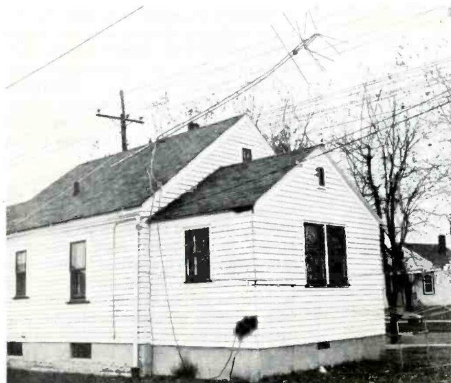
Fig. 15. Antenna That Fell on Utility Wires. Note Fire-Blackened Spot on House. (Courtesy NFPA.)
