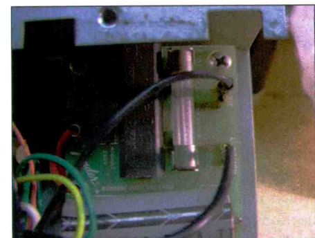
Figure 9. An internal fuse that would not be readily seen without removal of the chassis.
