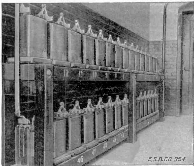
FIG. 1,662.—Portion of a battery room showing Exide battery installed on two tier racks. On account of the increased weight of the elements and the higher discharge rates required of the type cells shown, the plates are shipped loose and the cells assembled on the ground; the plates are first placed in the jars and then lead burned to lead bus bars. Bus bars used at the ends of rows are reinforced by copper bars embedded in the lead in order to provide ample conductivity to the terminal connectors.
