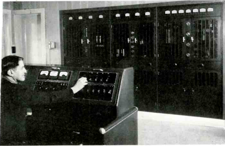
Chief Engineer Norris E. Grover puts the new 5 KW transmitter on the air.
