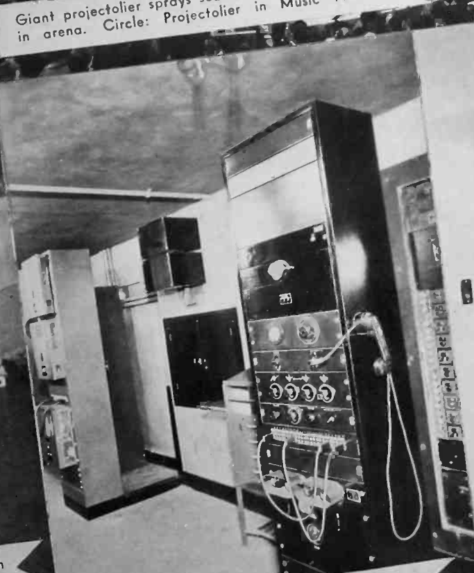
Combined panels containing public address and ERPI switching equipment and amplifiers
