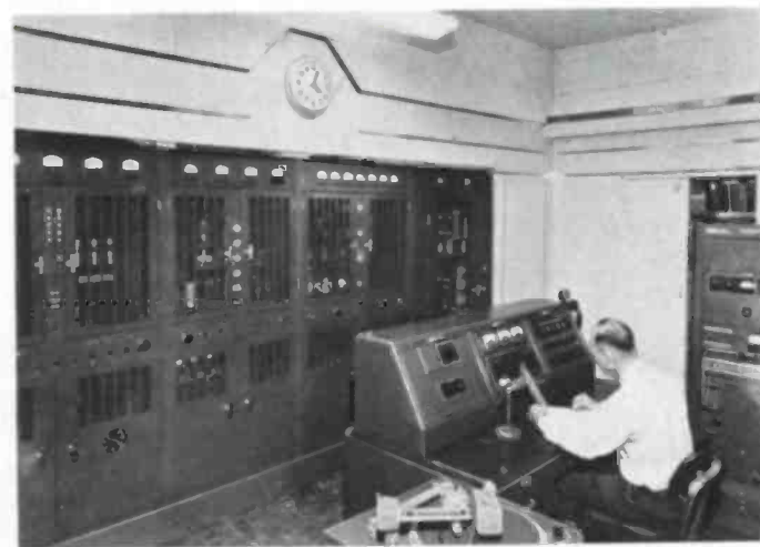
Control room, showing 5 KW AM transmitter, antenna control unit, control desk, and audio equipment at right.
