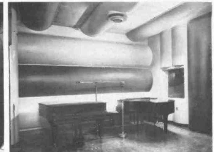
Polycylindrical wall treatment is used in large studio.
