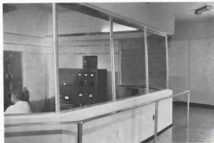
Public viewing lobby is separated from the transmitter control room by glass panels.
