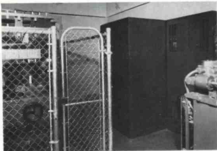
A chain link fence in transmitter room keeps personnel away from high voltage equipment.
