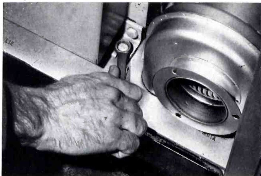
Bolted joints carrying current in transmitter must be kept tight to avoid vicious circle of resistance, heat, oxidation — more resistance.
