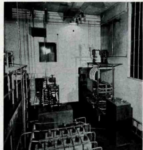
High-voltage area, rear of old transmitter, before units for new 50 were added. (See plan, page 37).
