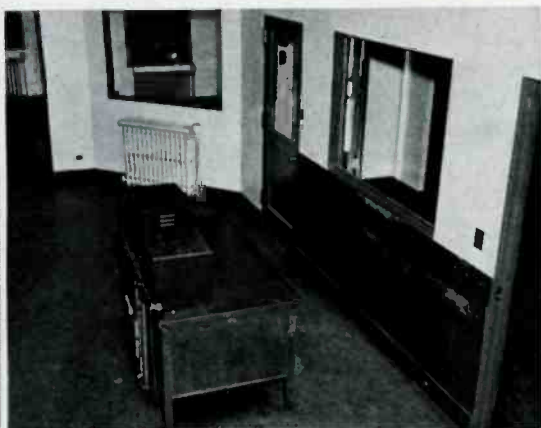
Above, control room before partitions were removed for new 50 kw equipment. In picture, page 24, the two 50 kw transmitters face each other in new room.
