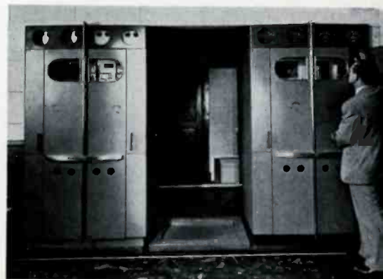
Top: THE NEW —WMGM's Western Electric 10 kw FM, beaming WMGM programs 7 hours a day to New York. At right is Grover Wizeman, transmitter engineer.
