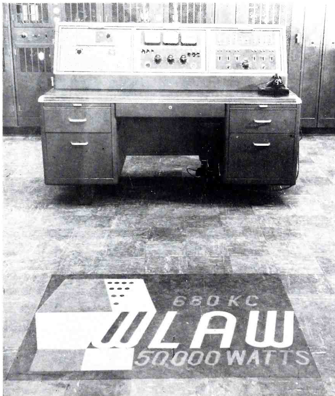
View of Transmitter Control Desk at WLAW's new 50 kw transmitter. New station facilities in the handsome transmitter building include line branching and phasing equipment with Western Electric 2A Phase Monitor at right of control desk and speech input equipment including a Western Electric 1126 Program Amplifier.
